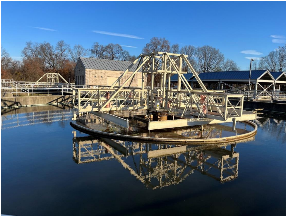
Fig. 19 – 2010 Infrastructure Project - Clarifiers
