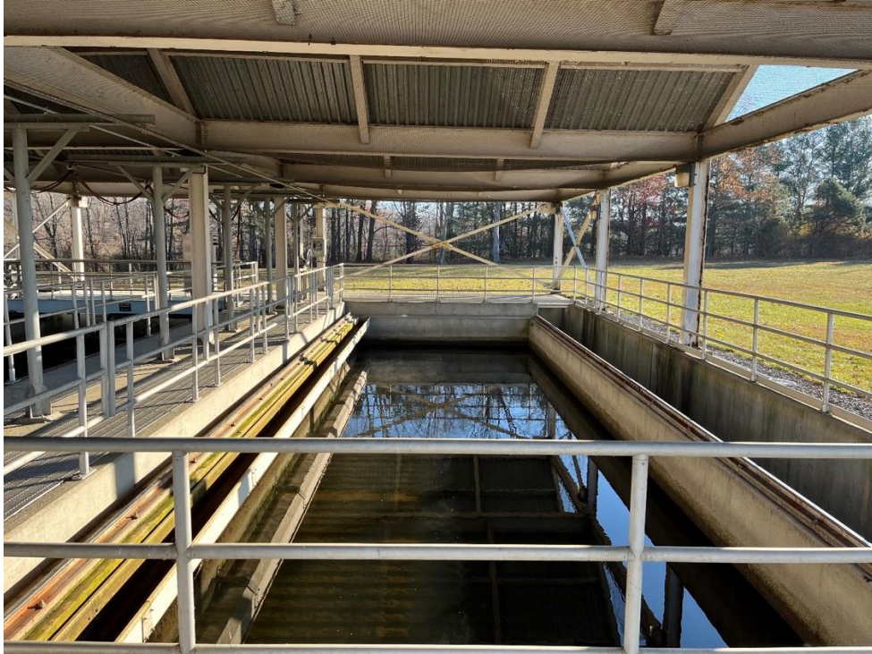
Fig. 20 – 2010 Infrastructure Project – Tertiary Filters
