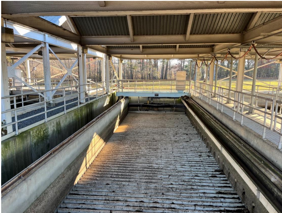
Fig. 20a – 2010 Infrastructure Project – Tertiary Filters
